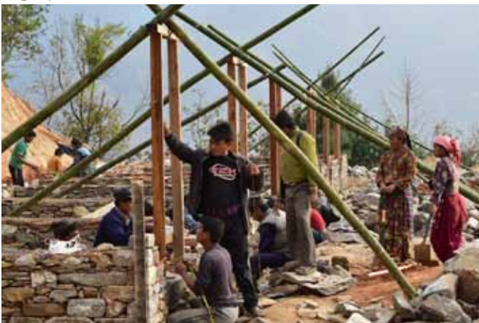
Local volunteers are building a new earthquake resistant school for the village.
