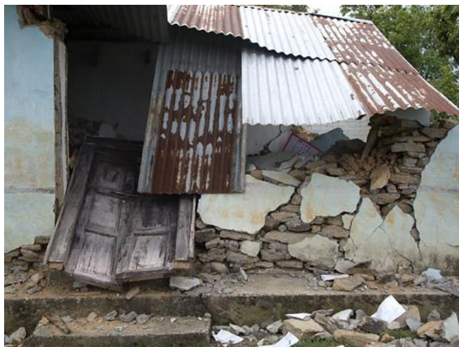
Destroyed Chupar school
